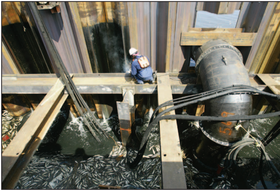
Dead fish in the floodwaters surround a worker as he repairs a levee in New Orleans.
